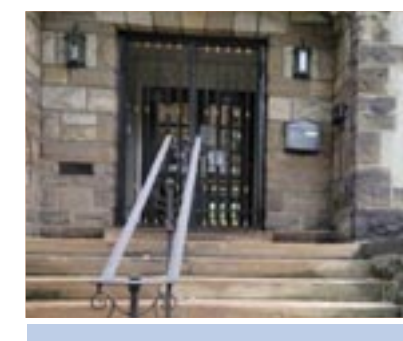
Restoration of historic door gates and the addition of a coordinating stair rail were completed in 2021.
